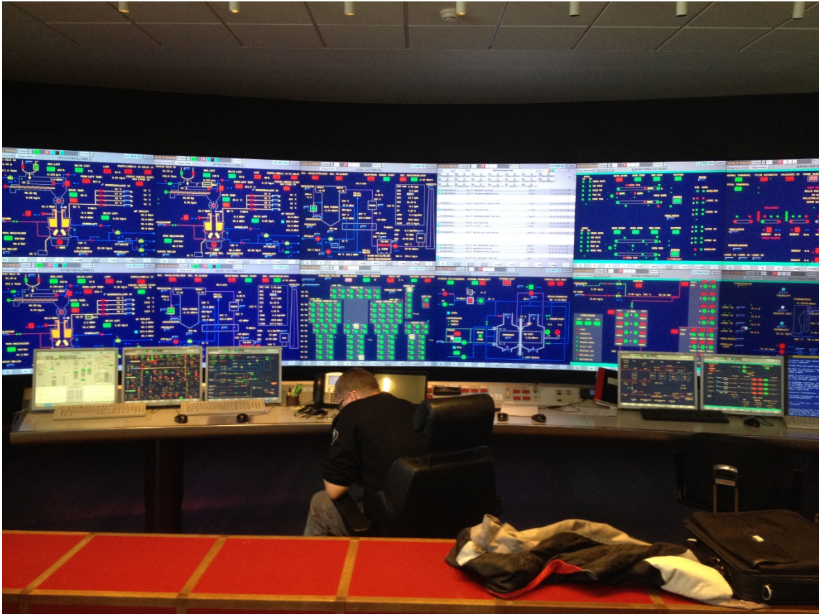
[3] Denmark, Copenhagen, Dong Energy power plant – control room
