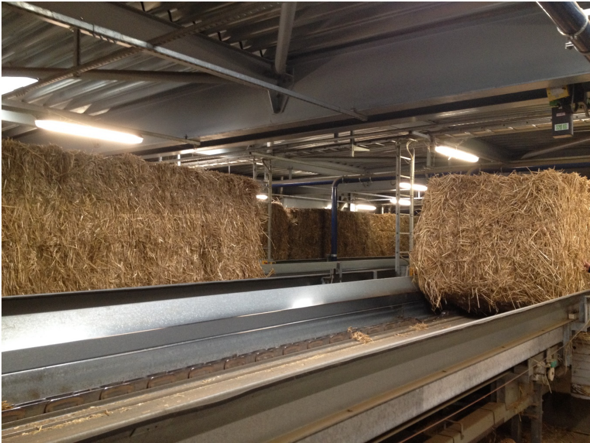
[4] Denmark, Copenhagen, Dong Energy power plant – biomass storage
