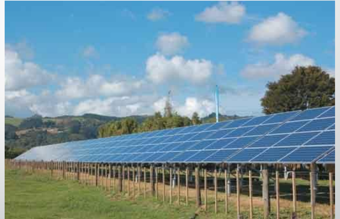
South Auckland Forging Engineering Ltd. (S.A.F.E. Ltd.) Solar Plant opened in Drury, 2012 360 PV Cells, 68kW (~476 kWh)
