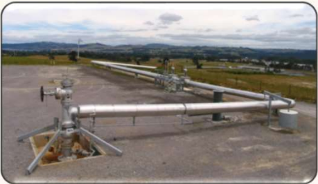
Production/ Injection Well
