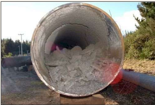
Silica deposit in geothermal fluid line (left) and steam turbine (below left / right)
