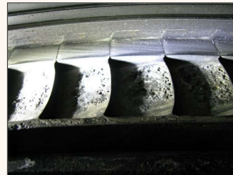
Corrosion on the diaphragm blades of a geothermal steam turbine
